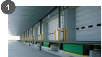
1 Car berths Sufficient number of car berths to enhance efficiency in cargo loading
