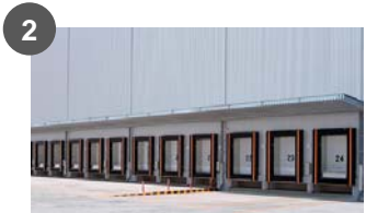
2 Dock shelters To prevent entry of outside air, rain, wind, moisture, dust, etc., during cargo handling
